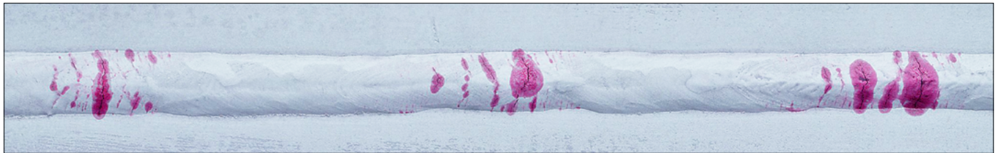
Crack indication with red dye penetrant on a weld seam
