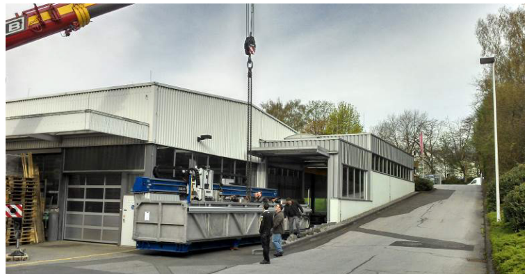
Figure 14. Readiness of shipment at the KARL DEUTSCH systems workshop in Wuppertal, Germany.
