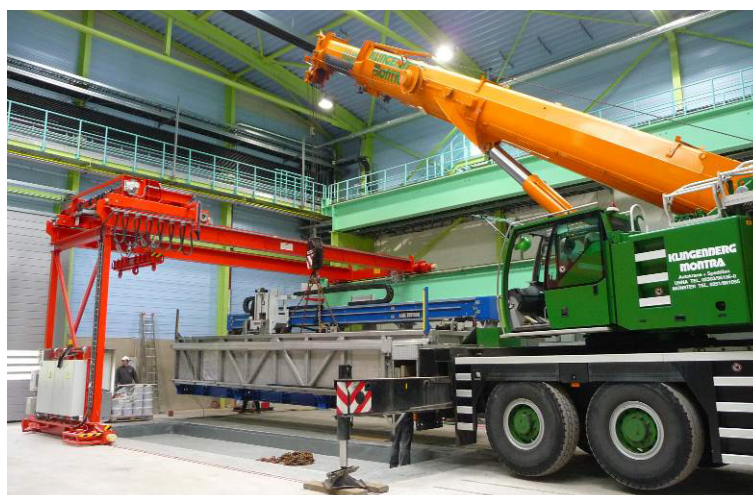
Figure 15. Onsite assembly at the VDM Metals GmbH workshop in the town of Unna, Germany.
